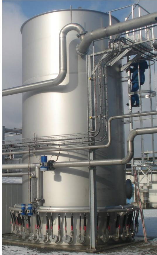
Figure 4: SMBF Biofiltration tank (3.000 PE)
